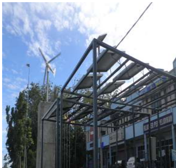
(b) PV array and wind power generation
